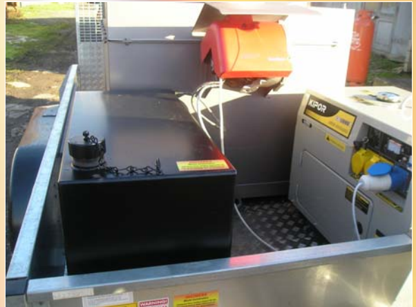
Fuel Tank & Generator
